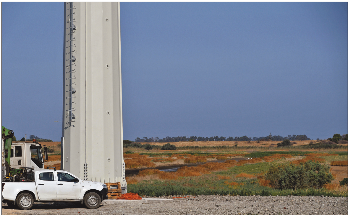
Figure 2. The power line structures and conductors will overtop areas where many species of birds take off, land, stop, feed, and breed (Lentini marsh July 26, 2022).
